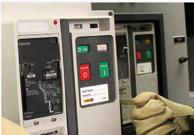
CIRCUIT BREAKER TESTING
